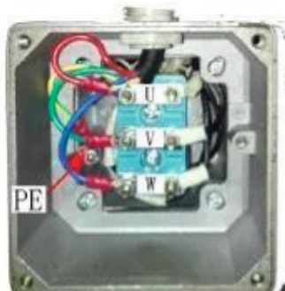
Motor wire connection
