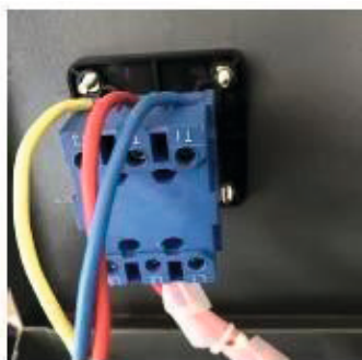
Power cable connection
